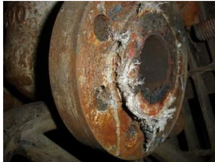
Damaged flange gasket
